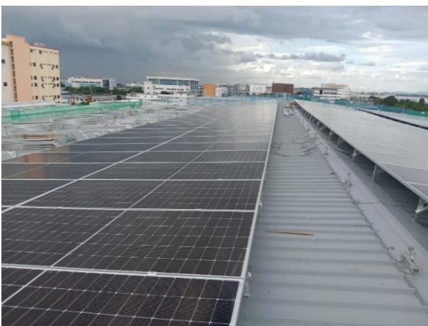
FYC - Solar panels
