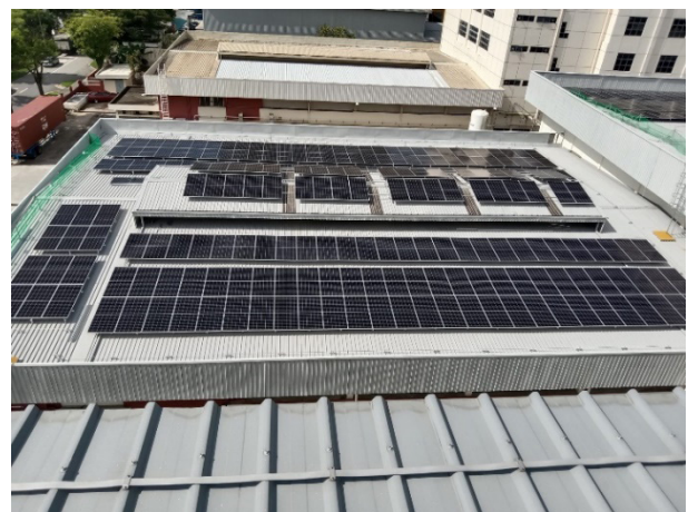
FYC - Solar panels
