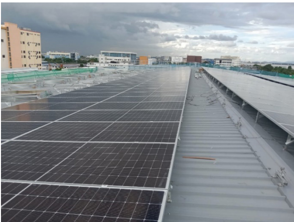
FYC - Solar panels
