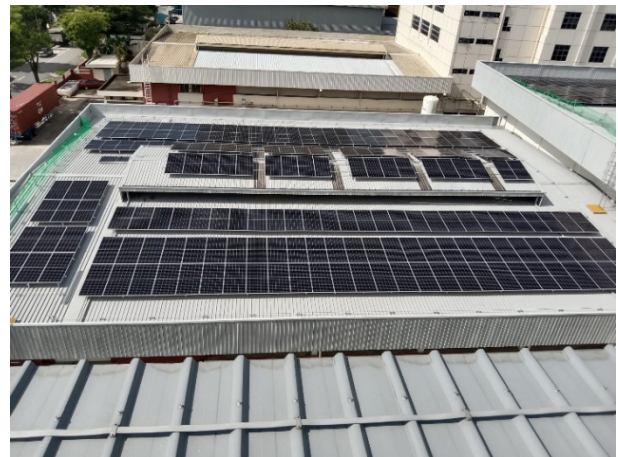
FYC - Solar panels
