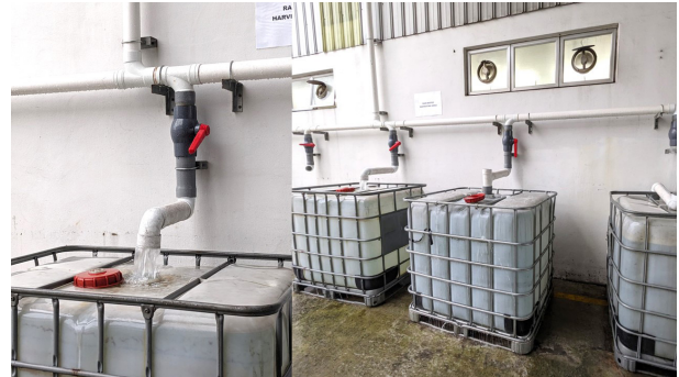
Water catchment for rainwater harvesting
