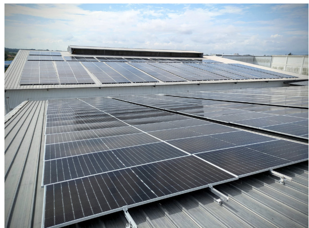
CA - Solar panels
