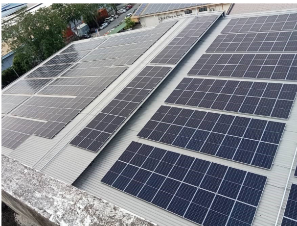
FHM - Solar panels
