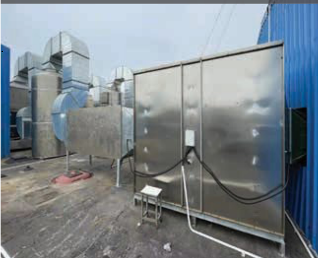
Spray paint workshop VOC treatment engineering
