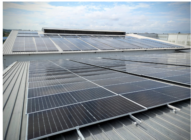
CA - Solar panels
