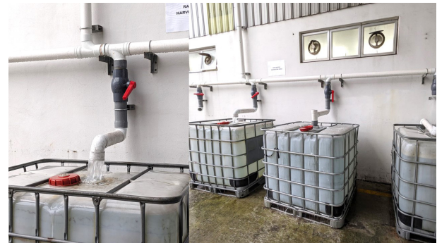
Water catchment for rainwater harvesting
